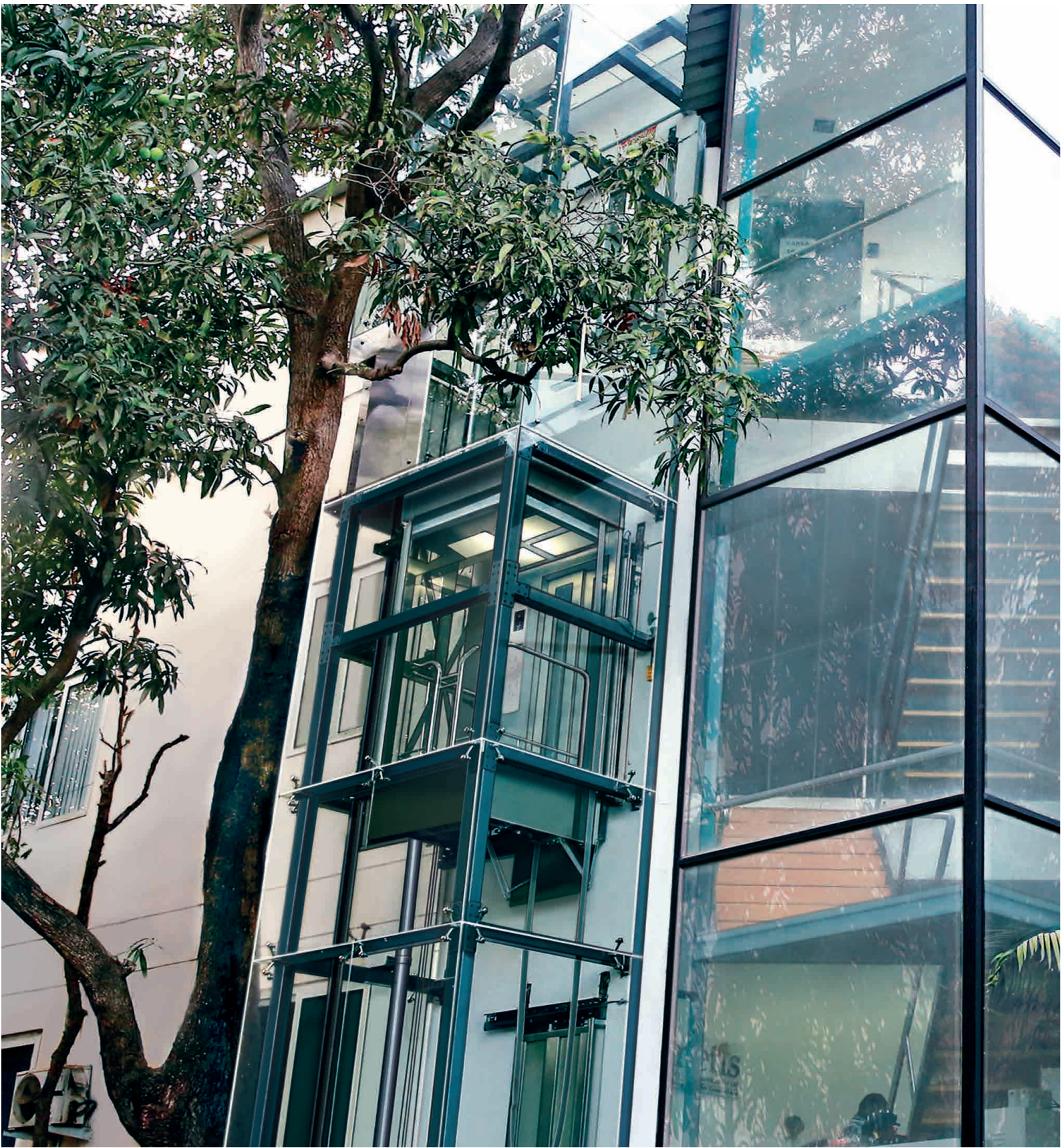
Installed at Karya Space, behind Hotel Woodlands
