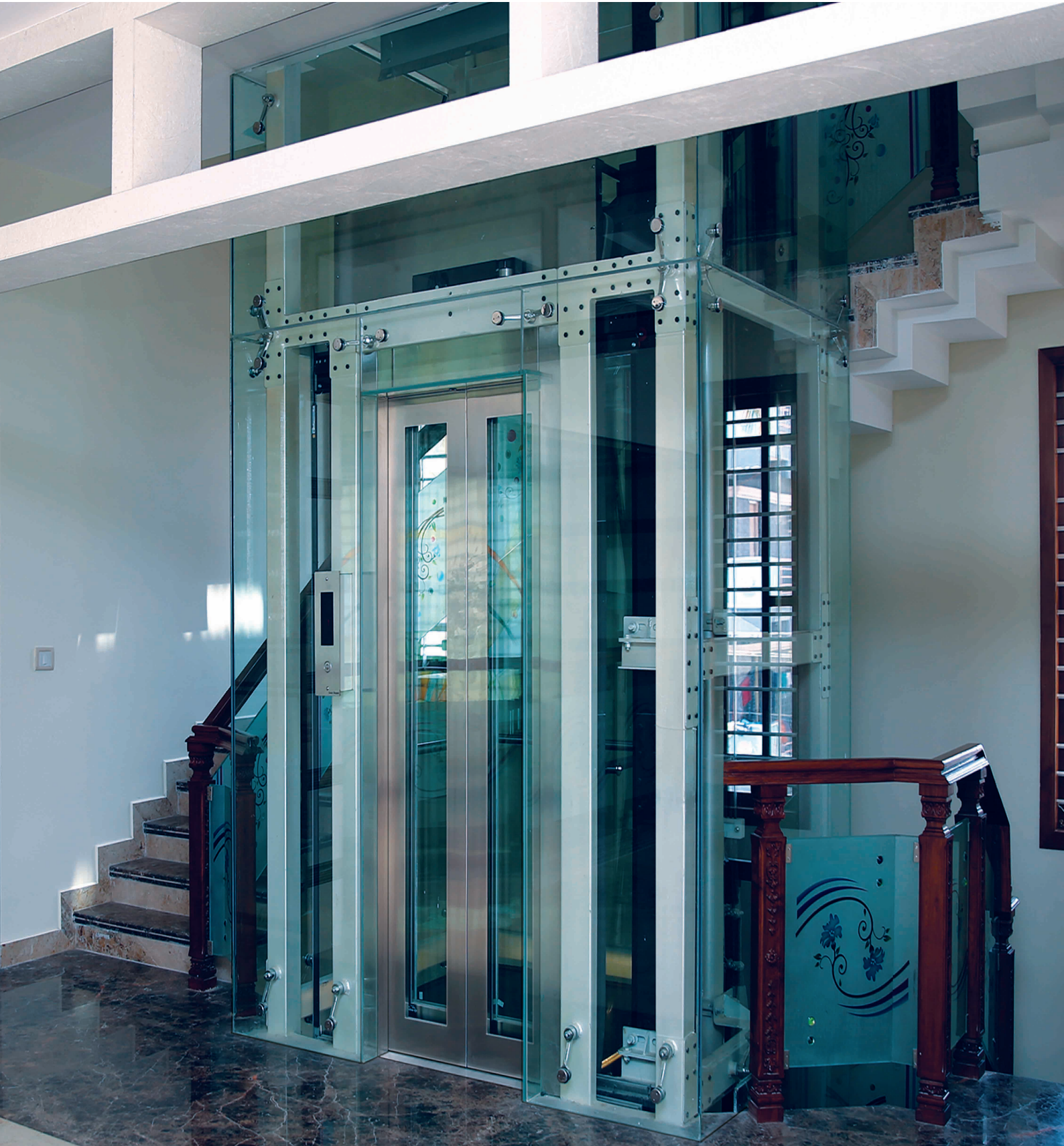
Installed at Mr. Ramamoorthy's House, Garudarcharpalya, near NIDHI Bakery, Bangalore
